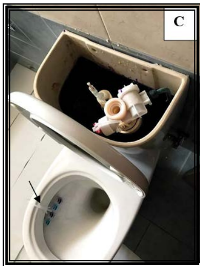
Figure 2c: Dye added to the cistern with cleaning aromatic balls in the toilet (C) drops not shown
